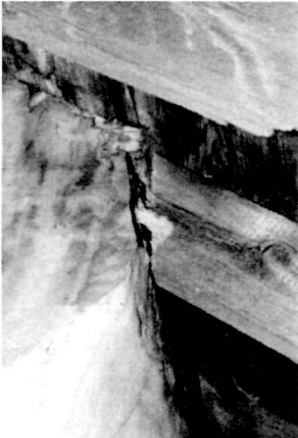
Figure 20 View of a rafter cut at the spiraling chimney of the Keeper's Dwelling, 1995.
