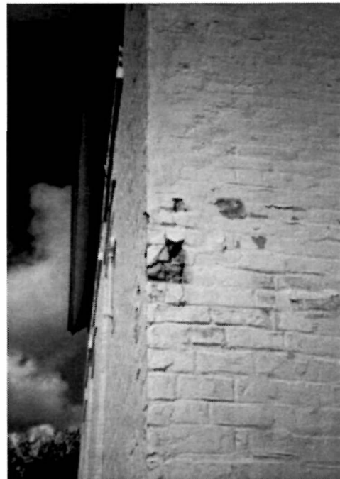
Figure 34 View looking west at the southeast corner of the Keeper's Dwelling, 1994. Note the deteriorated condition of both the cementitious parging and the underlying brick.
