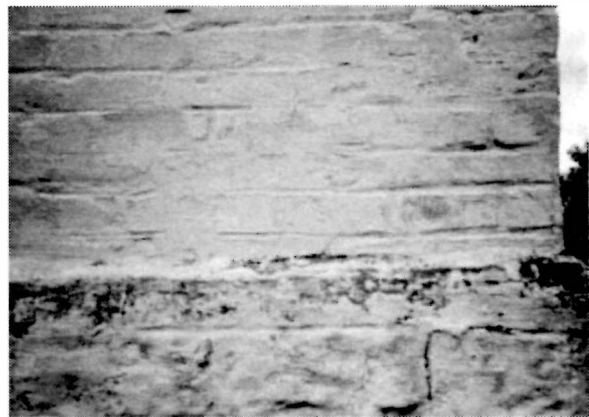
Figure 28 View of the west end of the north elevation of the Keeper's Dwelling, 1994. Note that the parging is crudely tooled to resemble mortar joints, a typical condition of the exterior brick wall surfaces.
