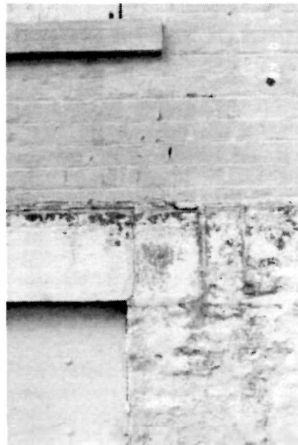
Figure 11 View of the east wall of the Keeper's Dwelling, south side, showing the window head stone cracking, 1995.
