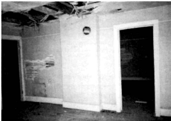
Figure 17 View of the south wall in the northwest bedroom (Room 204) in the Keeper's Dwelling, 1994. Note the rust at the plaster surface from the metal duct within the wall framing (at the bottom left corner of the photograph).
