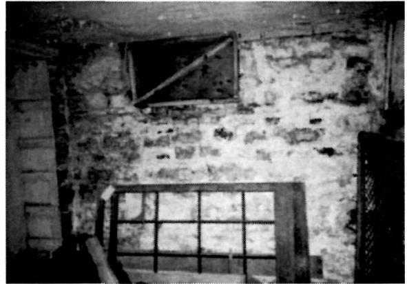
Figure 50 View of the east wall in the southeast basement storage room (Room B-01) of the Keeper's Dwelling, 1994. Note the remnants of the parging that was tooled to resemble masonry.
