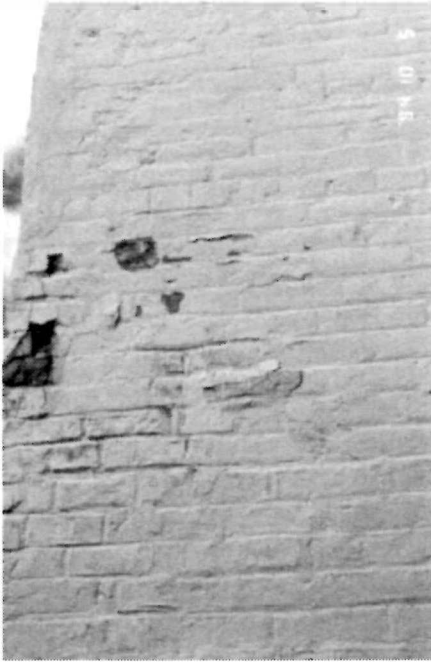
Figure 12 View of the east wall of the Keeper's Dwelling, south side, showing surface spalls near corner, 1995.
