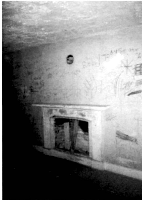
Figure 64 View of the fireplace along the north wall of the South Parlor (Room 104), 1994. Note that although the brick and plaster infill has been removed at this fireplace, the baseboard remains across the opening.
