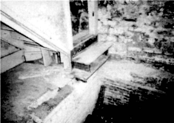
Figure 54 View of the stair that hangs precariously over the subcellar (Room B-03) in the Keeper's Dwelling, 1994
