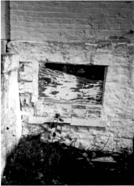
Figure 29 View of the basement window (D-1) at the east end of the south elevation of the Keeper's Dwelling, 1994. Note the deteriorated foundation wall between the window and the concrete steps.
