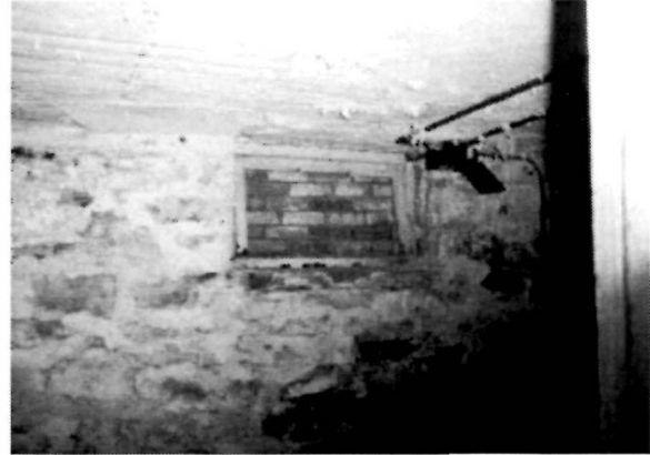
Figure 53 View of the east wall in the northeast basement storage room (Room B-03) of the Keeper's Dwelling, 1994. Note that most of the parging has worn or broken off of the stone wall surface.
