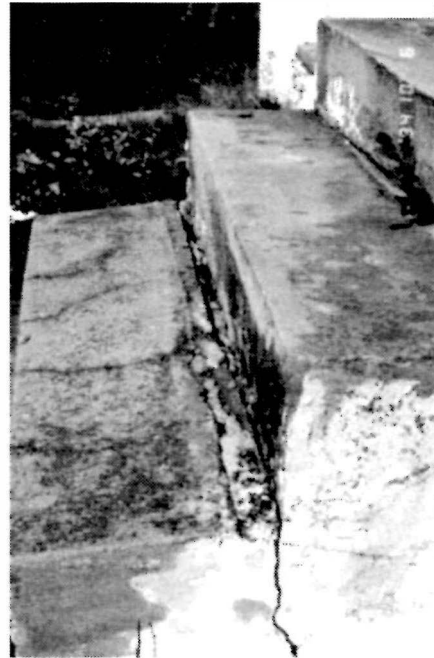
Figure 16 View of the stair distress at the south exterior stair of the Keeper's Dwelling, 1995.
