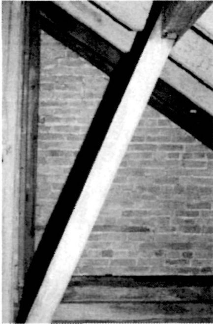
Figure 17 View of the diagonal strut and birds mouth jointing in the attic of the Keeper's Dwelling, 1995.
