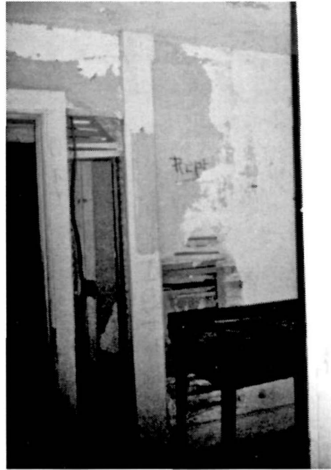
Figure 63 View of the west wall in the Keeper's Office (Room 102), 1994. Note the ghosted outline in the paint at the chamfered wood post, indicating that something was previously hung (and painted around) in this location.
