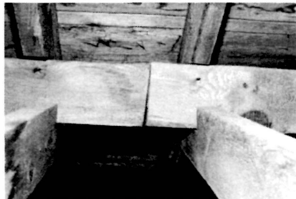
Figure 19 View of the beam butt joint at the south side of the roof, 1995.
