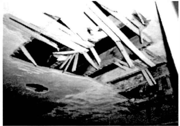
Figure 68 View of the ceiling in the southwest bedroom (Room 205), 1994. Note the large amount of missing plaster and broken lath, both the result of vandalism.
