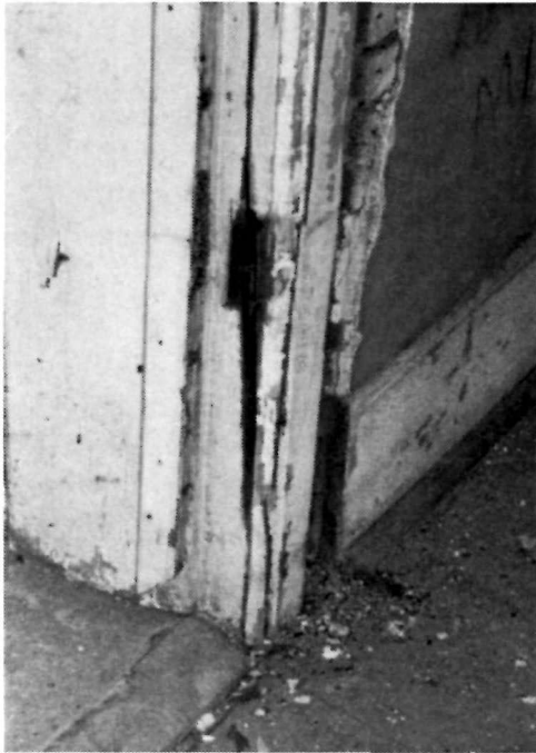
Figure 59 Detail view of the deteriorated and damaged wood door jamb at Door E-4 in Room 101 of the Keeper's Dwelling, 1994.
