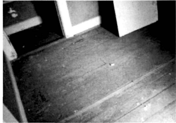
Figure 66 View looking southwest at the floor of the Stair Hall (Room 202), 1995. The heavy paint buildup has caused the paint to fail and loosen in large chunks.
