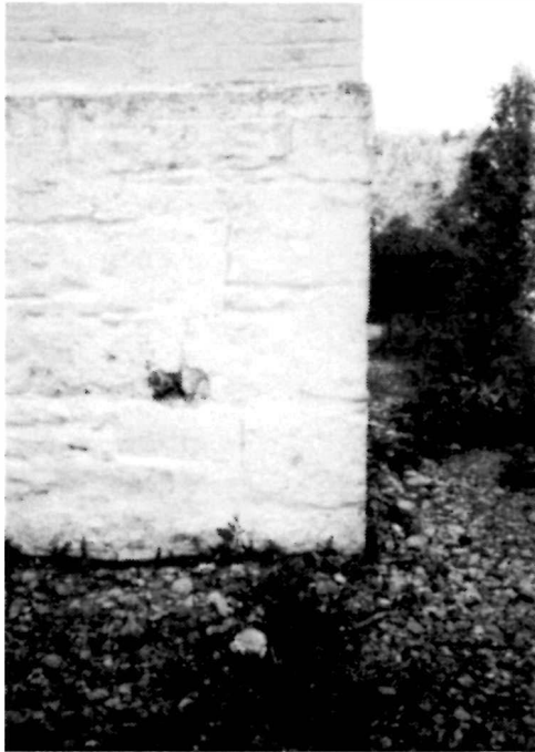
Figure 31 View of the northeast corner of the stone foundation wall at the Keeper's Dwelling, 1994. Note the cracking of the cementitious parge coat along the profile of the cut stone quoining.
