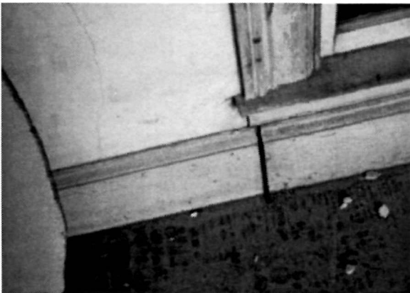
Figure 47 Detail view of the separating joint in the wood baseboard beneath a window in the Passageway, a typical condition beneath all four of the Passageway windows, 1994.
