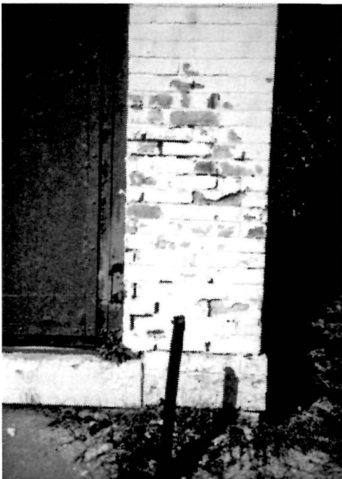
Figure 77 Detail view of the north end of the east elevation of the Brick Oil House, 1994. Note the spalling brick and deteriorated mortar joints.
