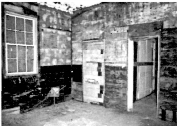
Figure 71 View looking toward the southwest corner of the east wing of the Fog Signal Building, 1995.
