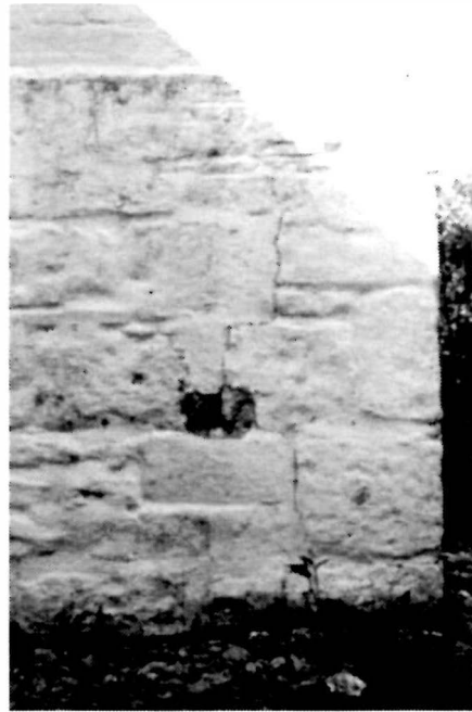
Figure 10 View of the foundation wall distress of the east wall of the Keeper's Dwelling, 1995.
