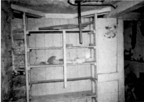
Figure 51 View of the south wall of the northeast basement storage room (Room B-02) in the Keeper's Dwelling, 1995.
