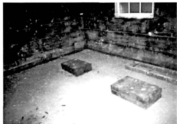
Figure 73 View looking toward the northeast corner of the Machinery Room in the Fog Signal Building, 1995. The concrete pads formerly supported two diesel generators.
