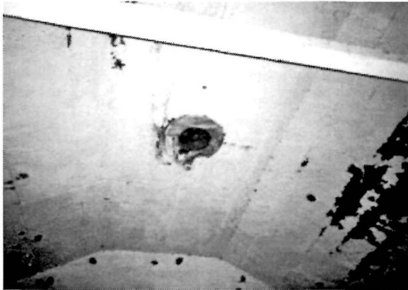
Figure 69 Detail view of an opening in the ceiling of the Fog Signal Building, 1995. A metal chimney stack once extended through this opening.
