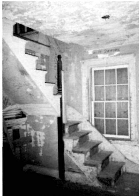
Figure 62 View looking northeast in the Entrance Hall (Room 101) toward the stair, 1994. Note that the balustrade and some of the tread nosing are missing at the stair, and the deteriorated condition of the adjacent plaster surfaces
