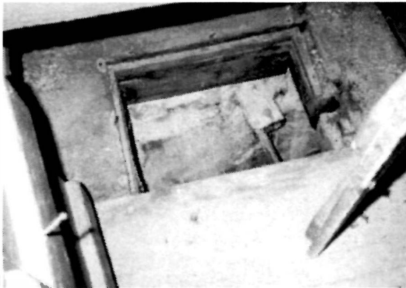
Figure 16 View looking down into the cistern located at the northwest corner of the basement of the Keeper's Dwelling, 1994.
