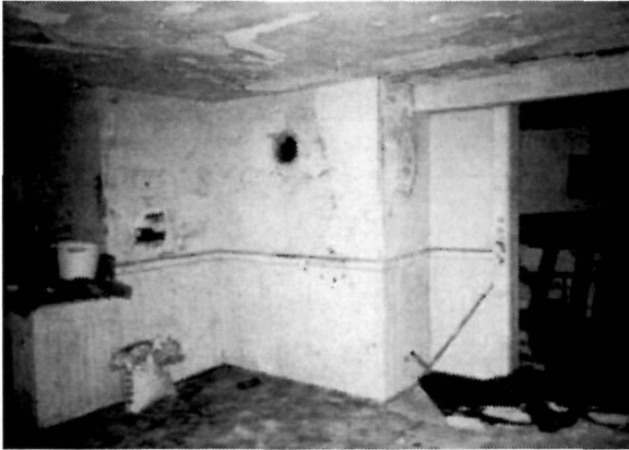
Figure 57 View looking northwest in the Assistant Keeper's Kitchen (Room B-06). Note the deterioration of the plaster at both the ceiling and walls.
